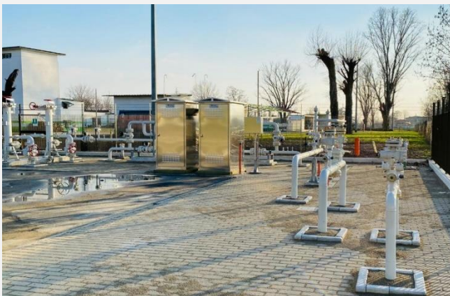
Attrezzature Green Fuel Company SpA
